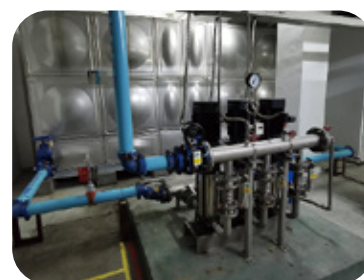
Secondary Water Supply
